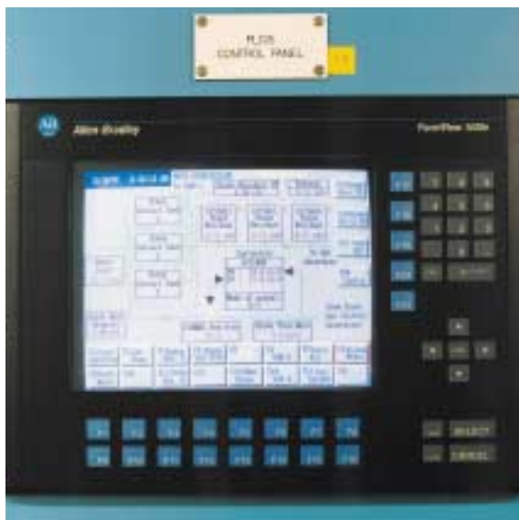
Figure 4: Control panel touch screen
