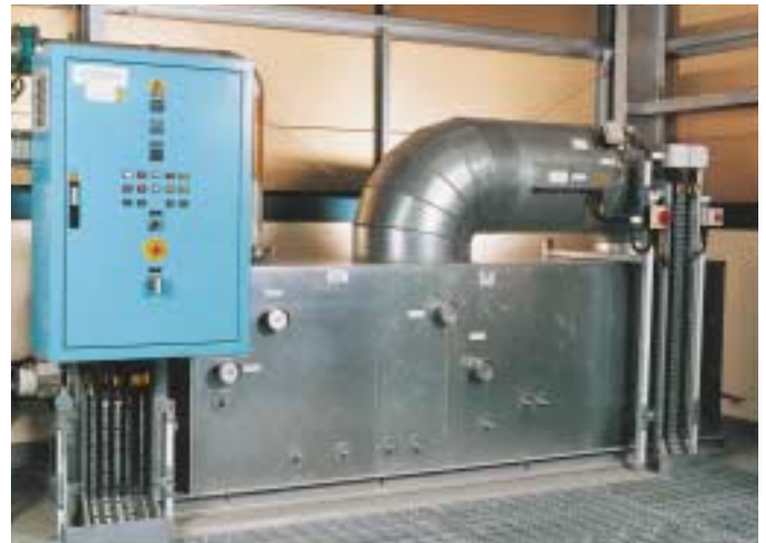
Figure 3: Vent ozone destructor and control box
